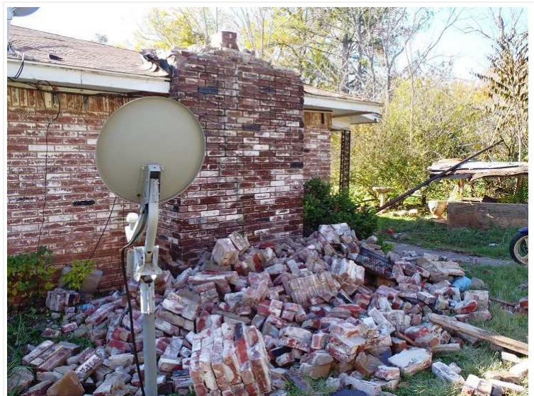
House damage in central Oklahoma from the magnitude 5.6 earthquake on Nov. 6, 2011. Research conducted by USGS geophysicist Elizabeth Cochran and her university-based colleagues suggests that this earthquake was induced by injection into deep disposal wells in the Wilzetta North field. Learn more about that research at: http://geology.gsapubs.org/content/early/2013/03/26/G34045.1.abstract . Photo Credit: Brian Sherrod, USGS.
