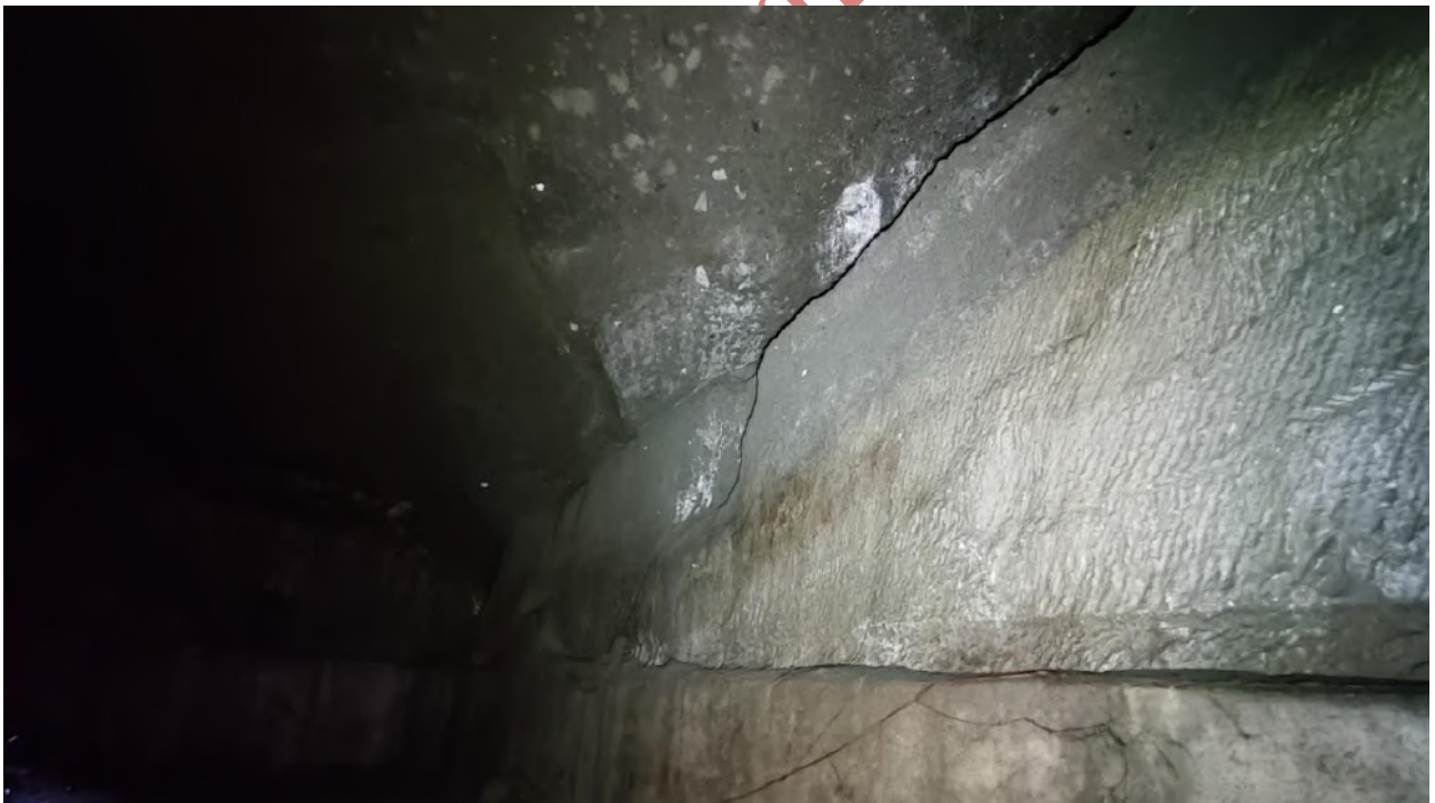
Fig. 8 - Hypogeum Area - South Wall. Presence of different types of masonry work and collapses of part of the stone ceiling and of the wall itself. Credits: Daniele Cataldi, Riccardo Bellucci, Settimio Tersigni, Marco Tudini.
