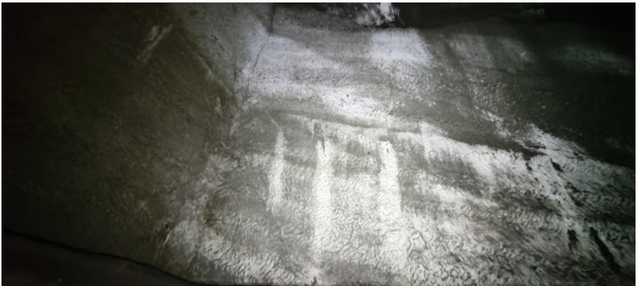
Fig. 11 - Hypogeal area - N and S perimeter structure. A large concretion of calcium carbonate is observed. Credits: Daniele Cataldi, Riccardo Bellucci, Settimio Tersigni, Marco Tudini.
